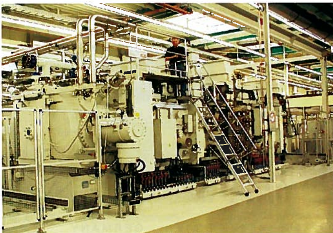
Fig. 1: Sequential vacuum hardening plant, throughput 800 kg/h
